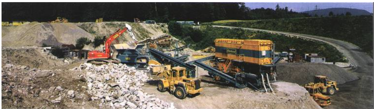
FIG. 5: Site for the production of concrete granulate from demolition material of buildings (before the ground was sealed and rainwater was collected and directed to a wastewater treatment facility)
